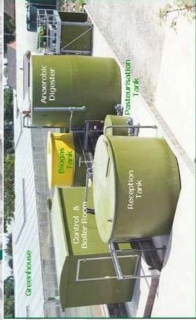
Biodigester facility : transformation of waste into energy
